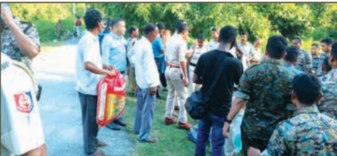
Execution of pipeline laying work in Jalpaiguri District, WB-II Section with the help of the police force
