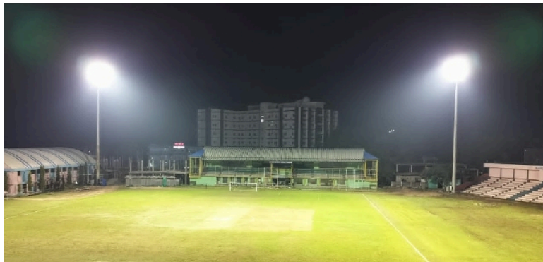
Fig. 3 Active Flood Lights at GDSA Stadium, Golaghat
