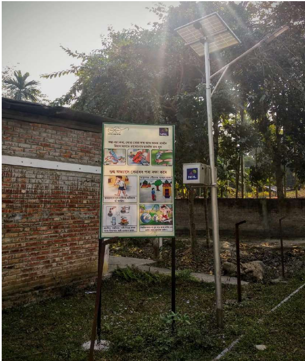
Image 4 Solar street lights
