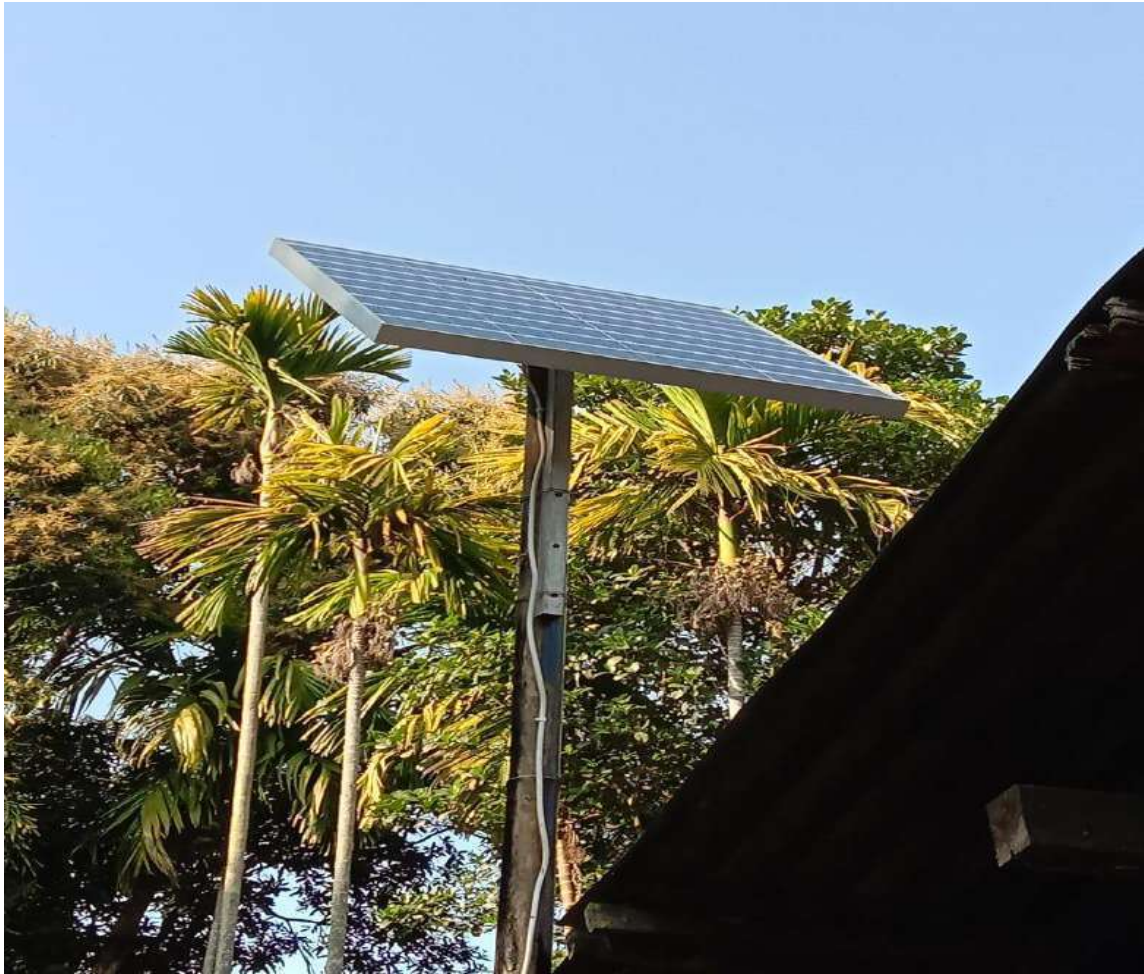
Image 3 Solar street lights
