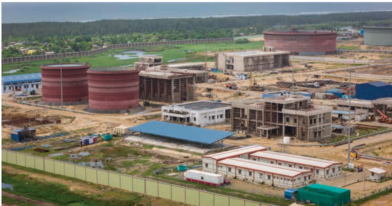
Crude Oil Import Terminal, Paradip
