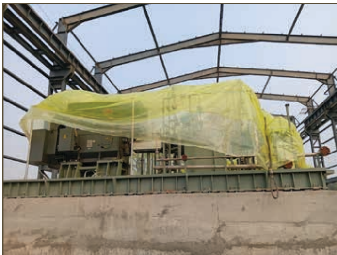
Centrifugal multistage mainline pump at IPPS-3, Mangaldoi
