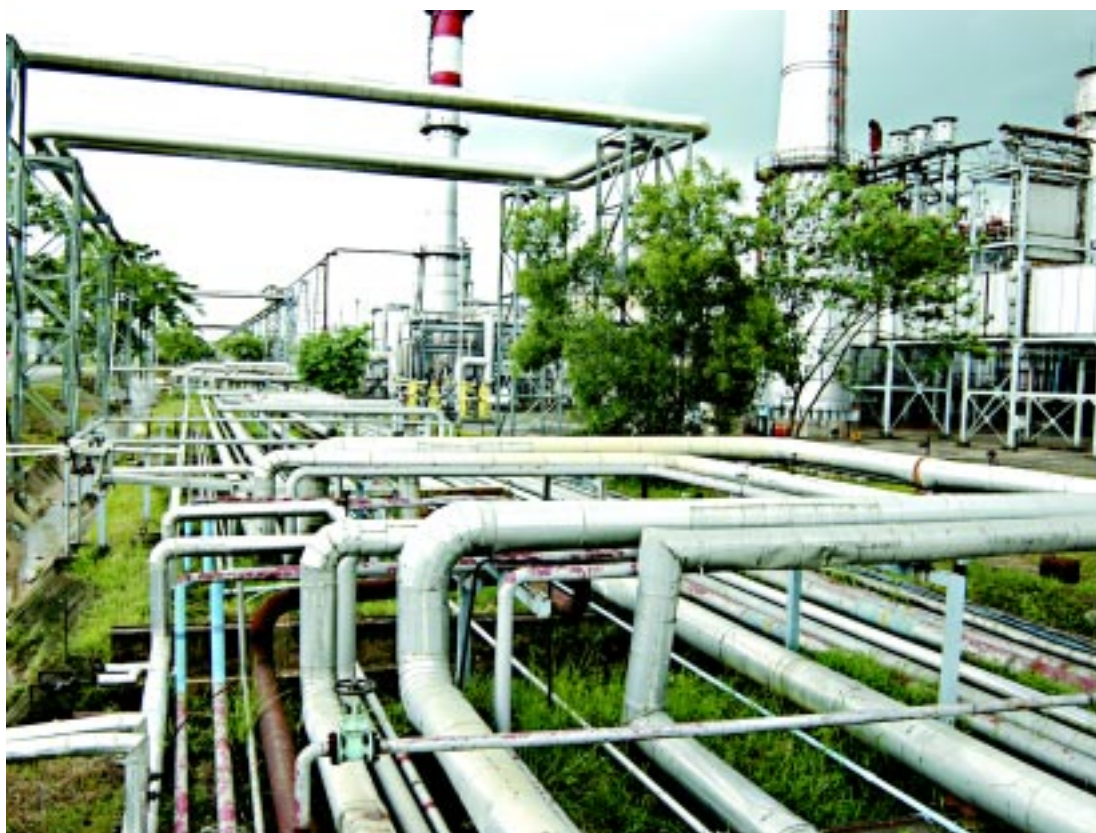
Pipeline network at Refinery
