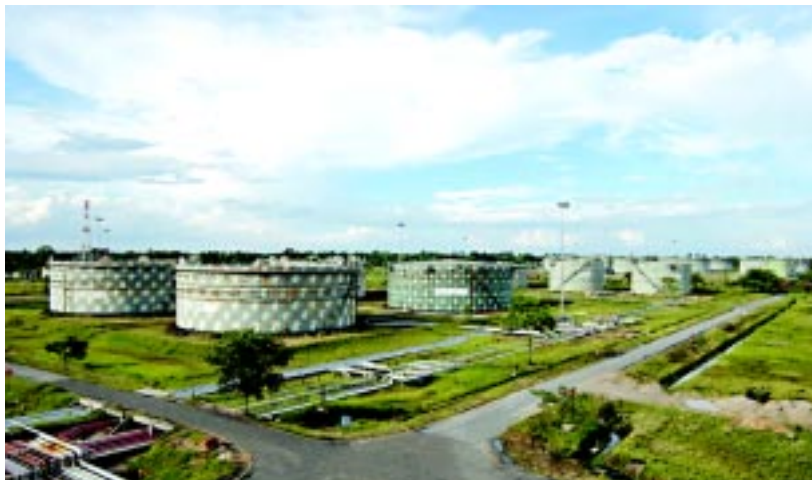
Product storage tanks
