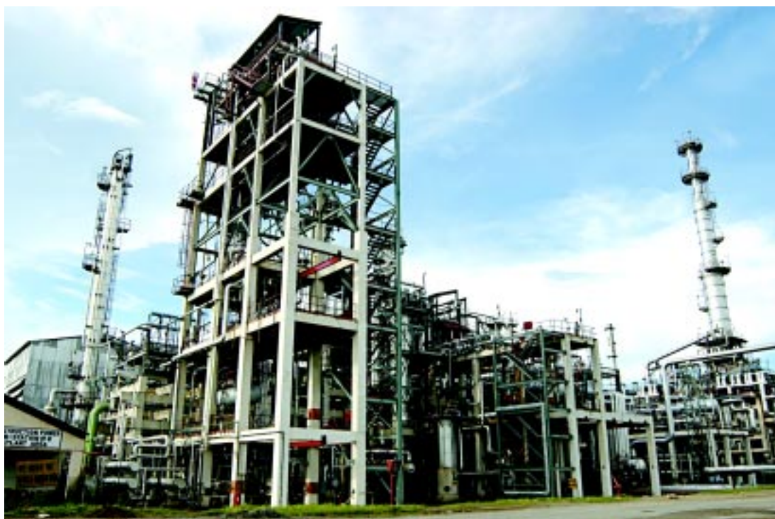
Fired Heater of Motor Spirit Plant
