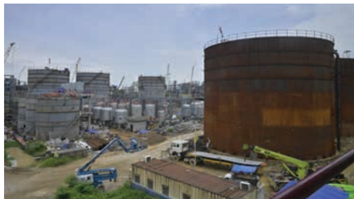
Demineralised Water Plant & Condensate Polishing Unit
