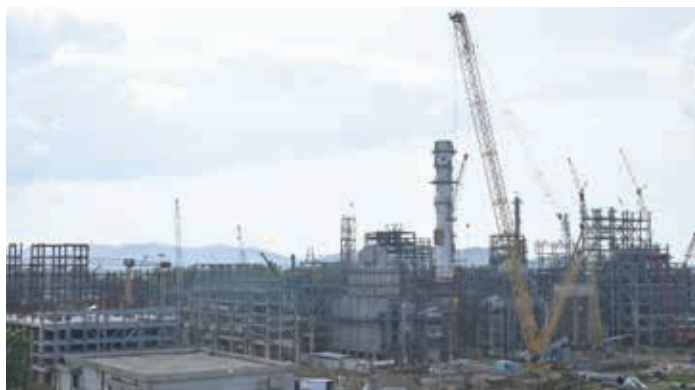
Crude Distillation Unit/Vacuum Distillation Unit
