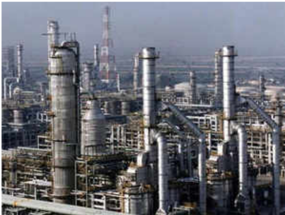
The expansion project involves setting up crude oil pipeline from Paradip to Numaligarh
