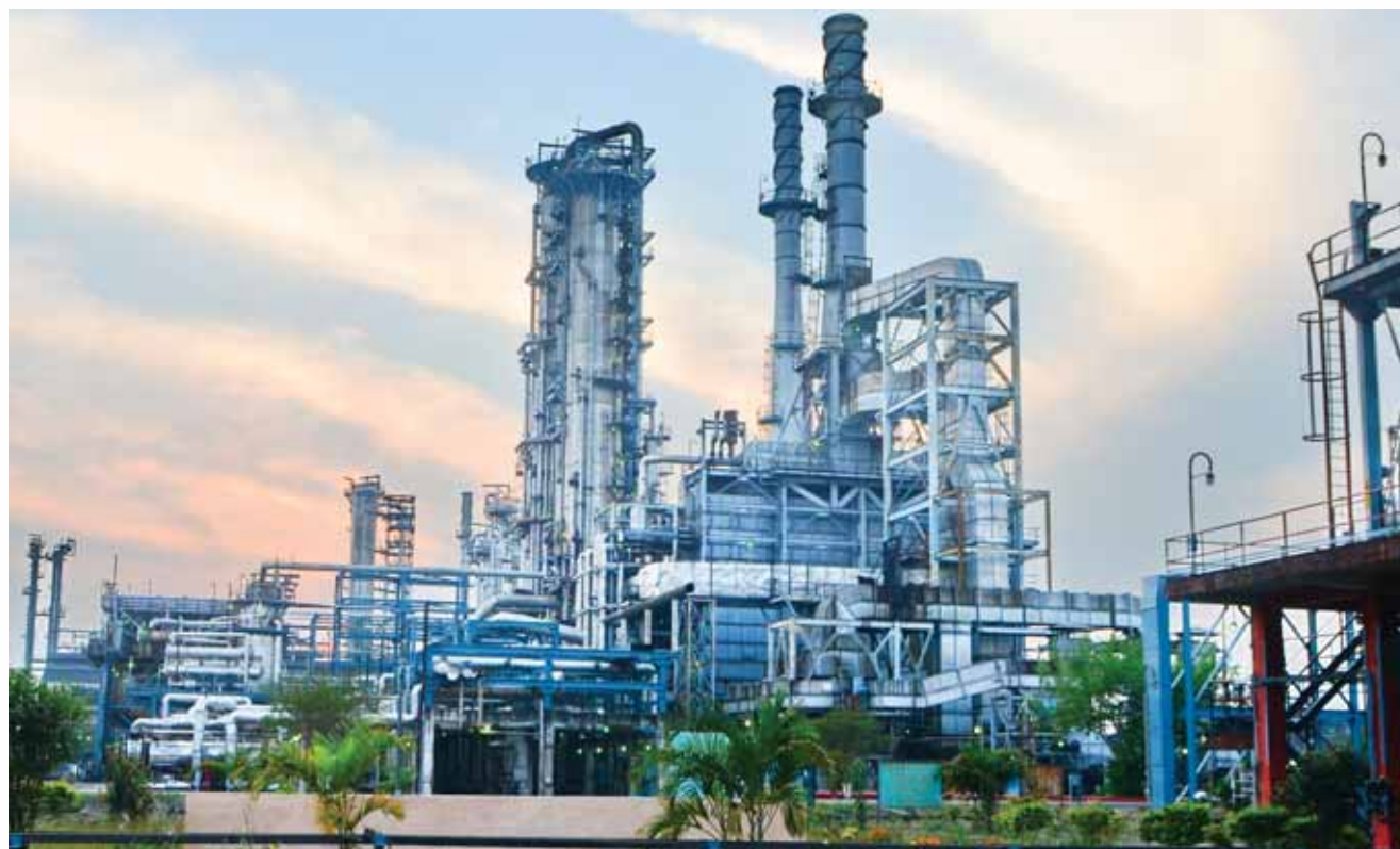
A view of CDU/VDU Unit
